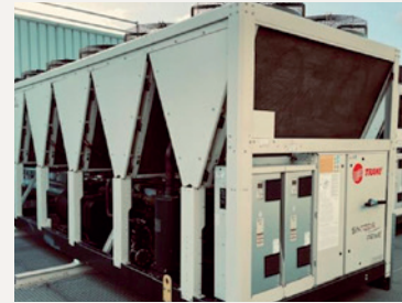
Replacement of process positive cold production - 2022
